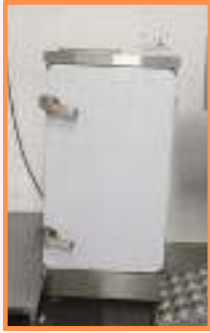
Installation of Idli-making machine in the School Mess.
