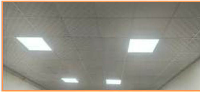
Installation of false ceiling along with LED panel lighting in all class rooms and labs.
